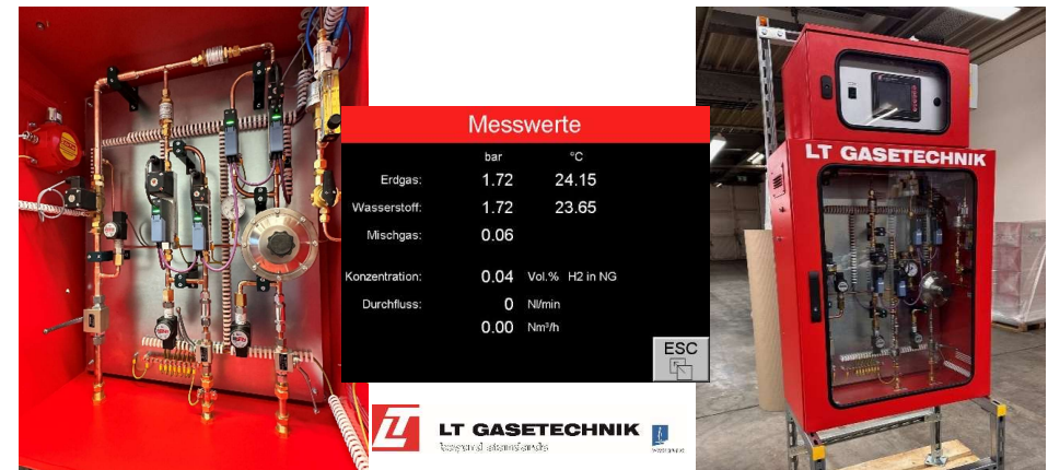
gas mixing station
